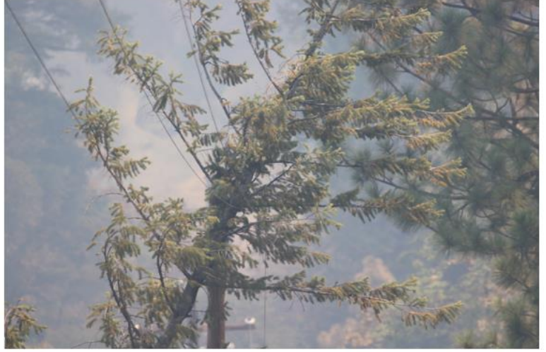
Douglas Fir Tree leaning into PG&E's Lines
